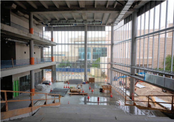
Construction of a new building as part of the redevelopment of the Northwest campus.
